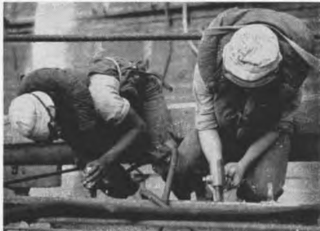
SAFETY-CONSCIOUS CHIPPERS are lashed to their staging, wear goggles to protect eyes from flying chips of paint. Pulled-down bats protect hair.
