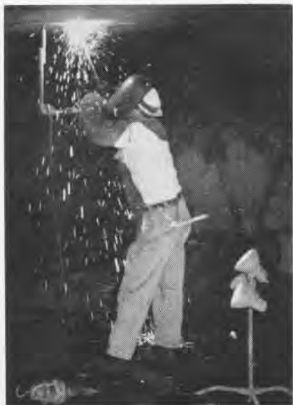
A CIVILIAN WELDER closes a hole in the hull, cut for access to obscure voids.
