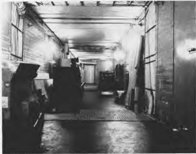
PASSAGEWAY of connected modules at Eights Station shows the roominess of the small units. It is viewed here while being constructed.
