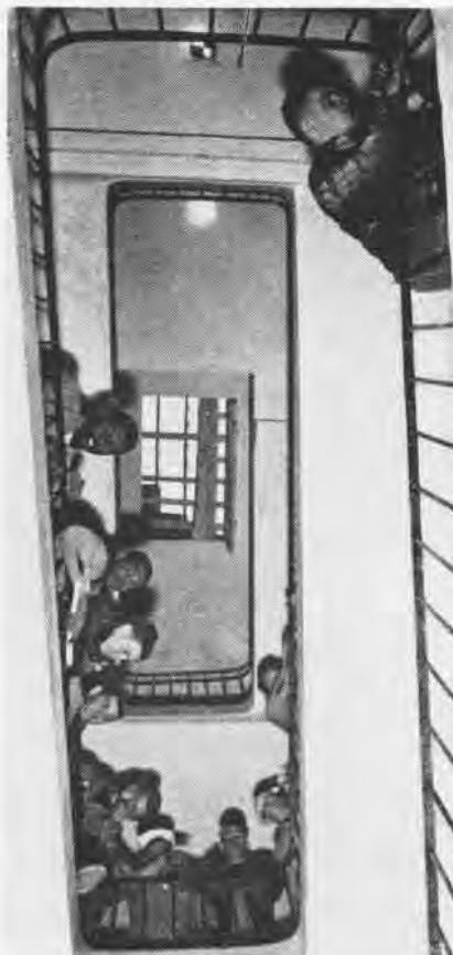
SHANG's Air Department renovates the staircase in a Cannes, France, home for the aged.
