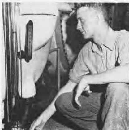
WATER LEVEL in No. Two evap is regulated by C. E. Lindsey, FN, as part of his duties.
