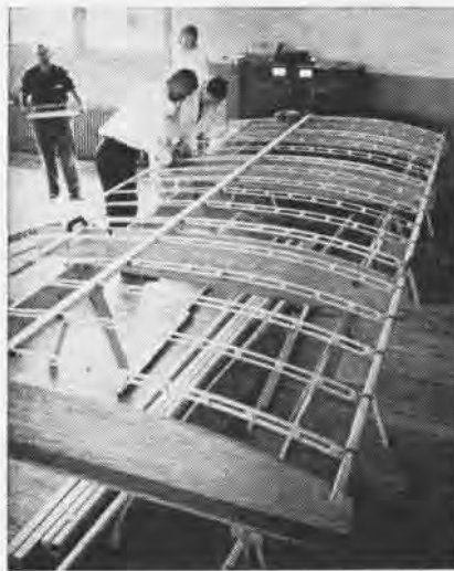
WINGS FOR the airplane were built in Hobby Shop at NATC; here one panel is assembled.
