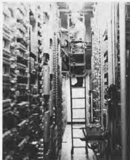
THE SPECIALLY designed telephone communications equipment is vital to ATC operations.
