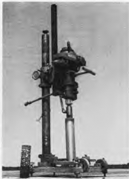
PAVEMENT CORE drill is cooled by water and penetrates runway surface in minutes.
