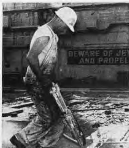
DUE FOR replacement, flight deck planking is removed from Oriskany by worker.
