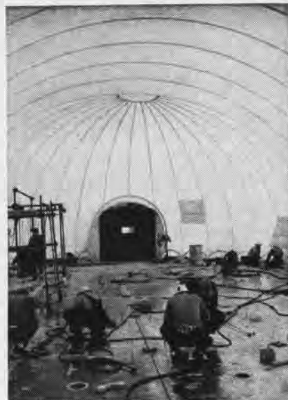
WORKERS under nylon "bubble" on flight deck of Shangri La secure new planking.
