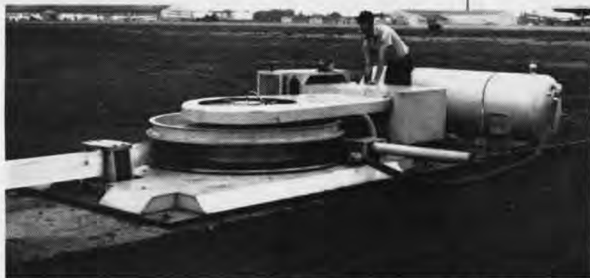
AT NAS ATSUGI, Japan, in May, a newly installed E-28 rotary hydraulic arresting gear was tested and certified for use. The E-28 has a greater capacity for engaging aircraft and a faster retraction than the two E-14 units located at either end of the runway. A twin-engine prop plane, the C-1A, was used to test the new recovery system, located at the midpoint of the runway. The aircraft "hit the gear" at a speed of 115 miles per hour.
