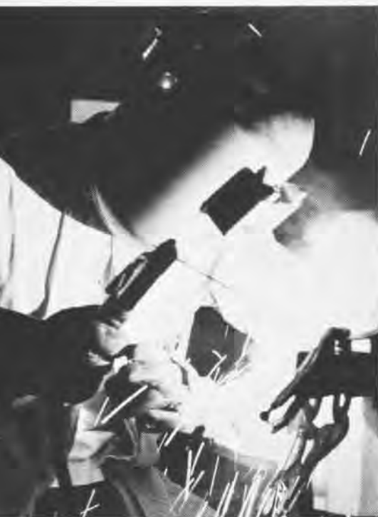
A SHIPFITTER aboard USS America uses an arc weld to repair a bracket on a bunk. The metalsmiths say they can fix anything.
