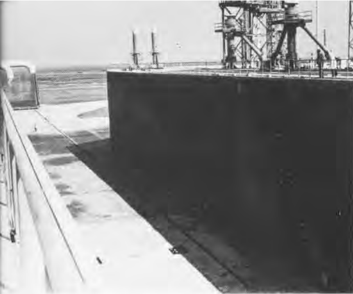
At launch time, huge flame deflectors move into position in this trench. Permanent pedestals on pad's surface cushion mobile service launcher during liftoff. Note man in left center.
