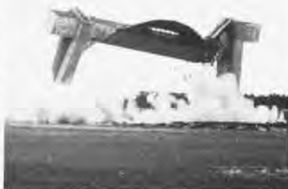
Blimp hangar pylon comes tumbling down.
