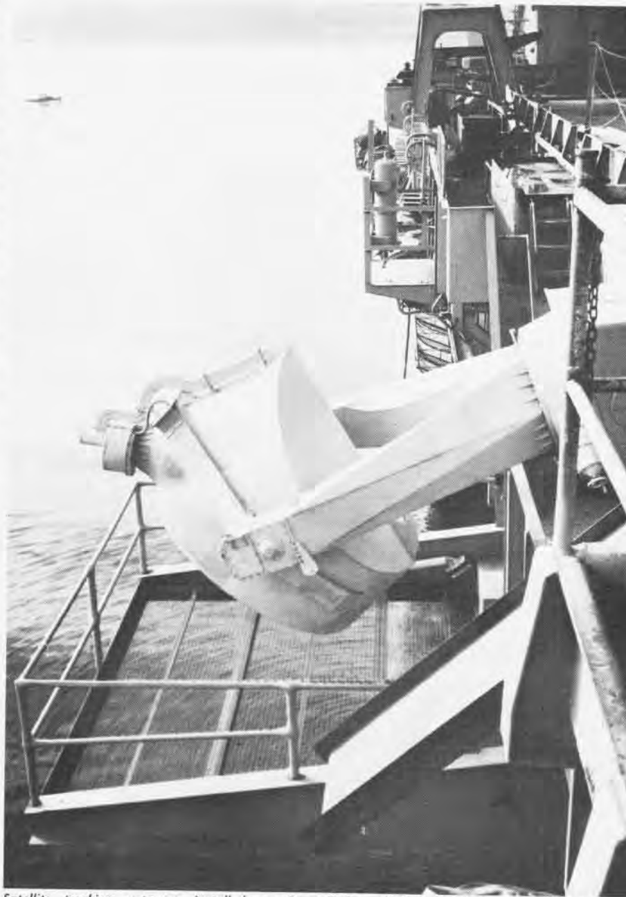
Satellite tracking antennas installed on Constellation eliminated shipboard interference.
