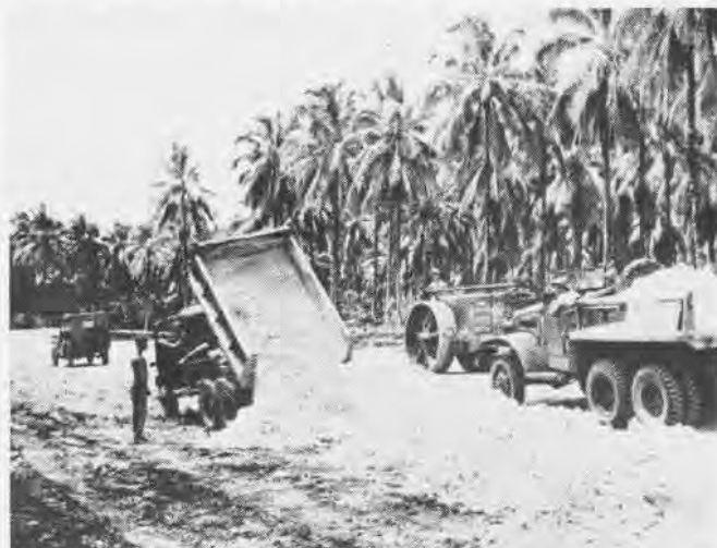
6 Operating on a round-the-clock schedule, Seabee trucks haul in crushed coral for placement on the taxiways and hardstands as the airstrip comes down to grade. Power roller nearby will flatten coral into smooth surface for the fighters soon to arrive
