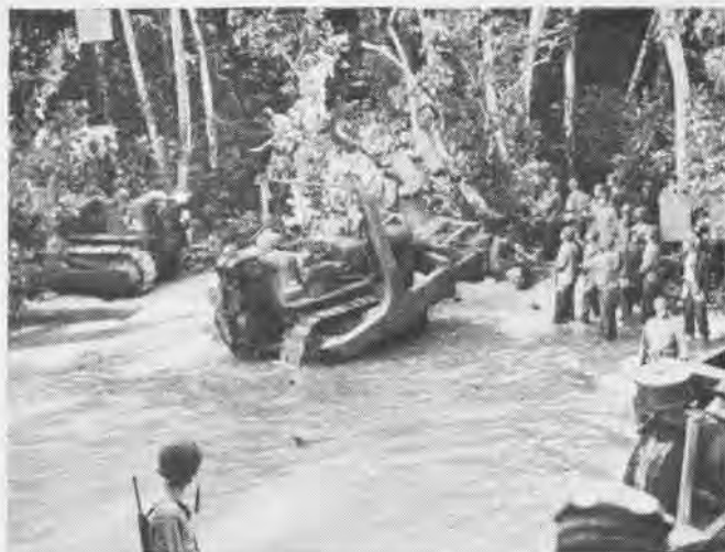
1 As soon as LST nosed up to shore, the ever-present Seabee bulldozers went ashore to push back the steaming jungle so supplies could be landed on beach. Note 20 mm. gun mount on blade of right-hand bulldozer, which later was set up on shore
